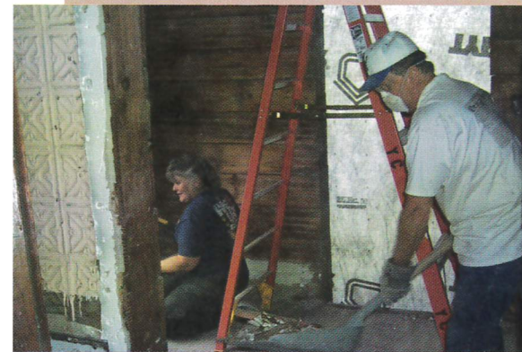
President Wayne and Darlene Baker joined forces with the Sojourners in the many renovation projects that took place over the summers.
